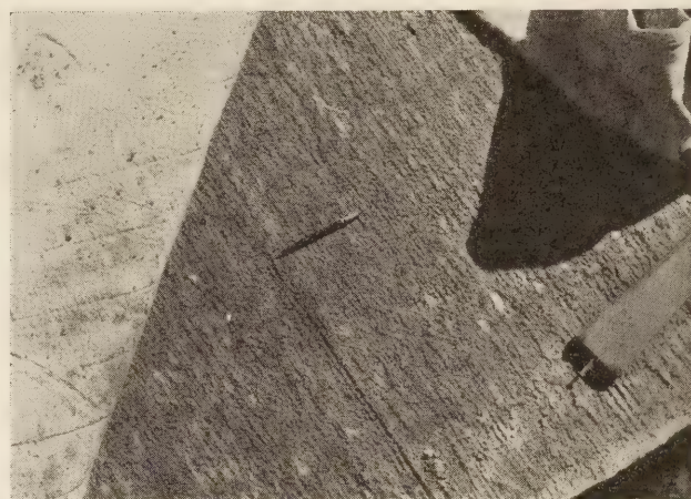
FIGURE 3.—PORTION OF CONCRETE PAVEMENT SLAB AND COTTON MATS USED IN CURING IT.
